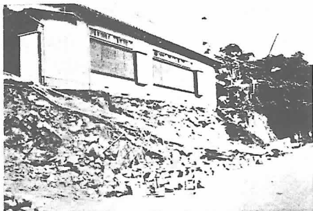
Fig. 1c. Collapse of a masonry retaining wall at Ikadaba, Kawazu-machi.
